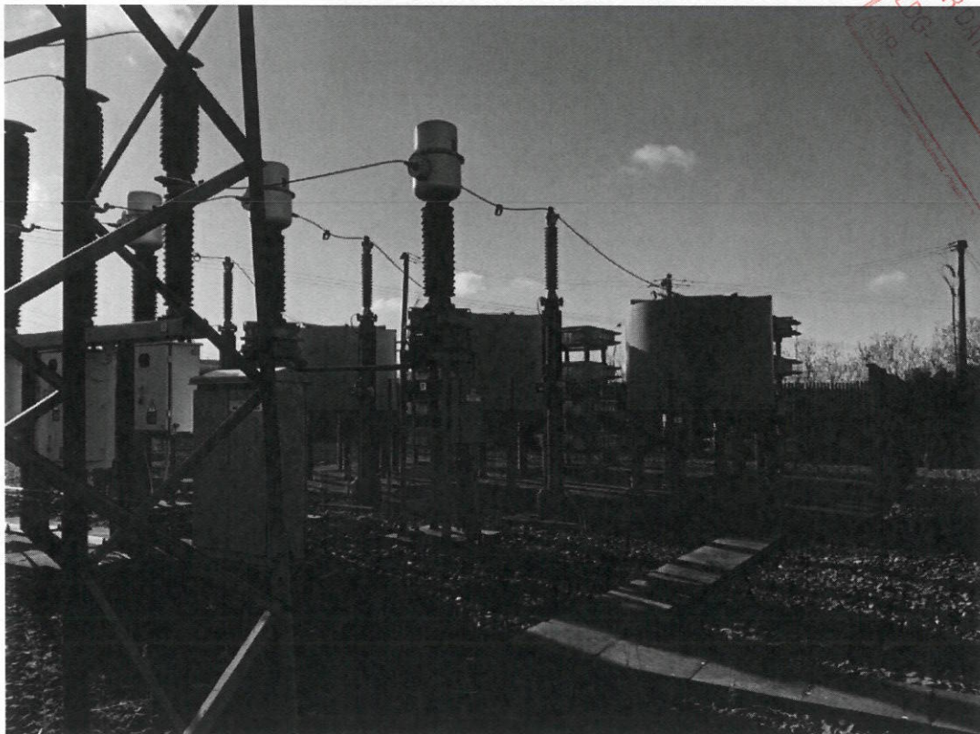
Figure 3: Photo of similar infrastructure as planned within an existing substation.
